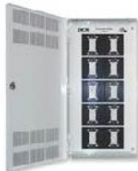
Lighting control panels
